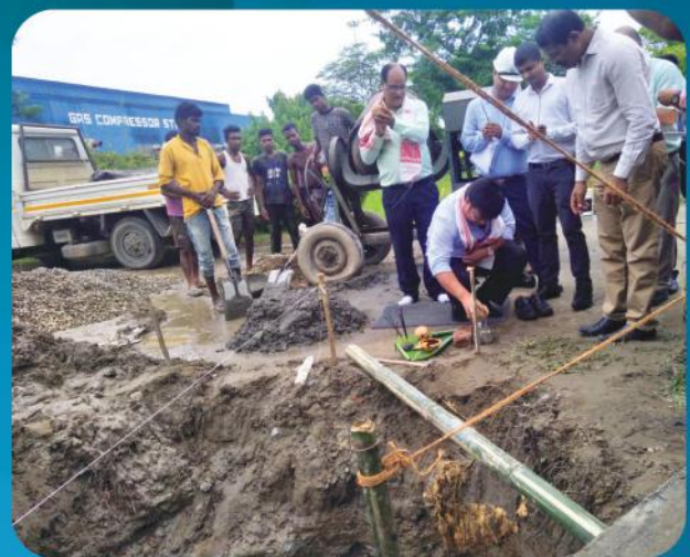
Laying Foundation Stone for 1st floor of office building construction at DS, Madhuban by MD, AGCL & Addl. Director, DNPL.
